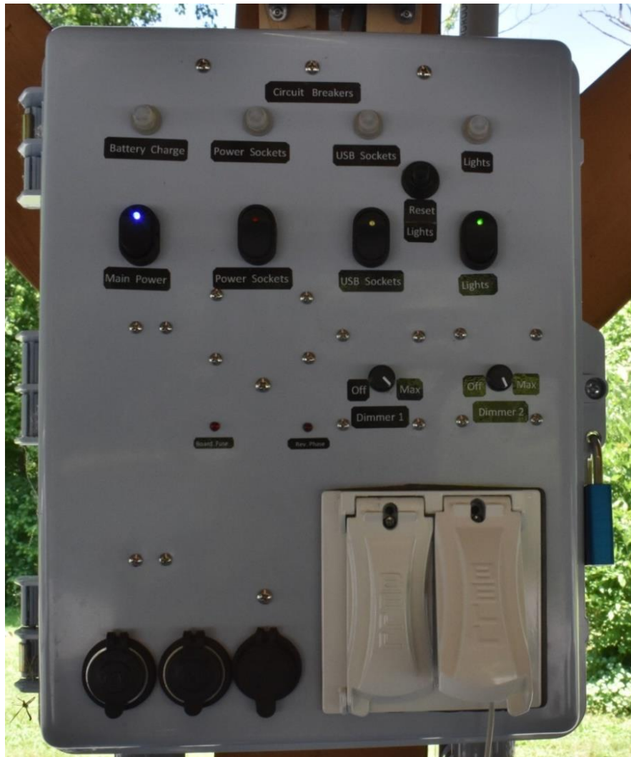
Figure 5. Solar Power Distribution Panel
